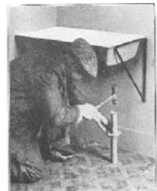
Figure 7: Lead pipe should be flanged to fit the pipe clamp.
